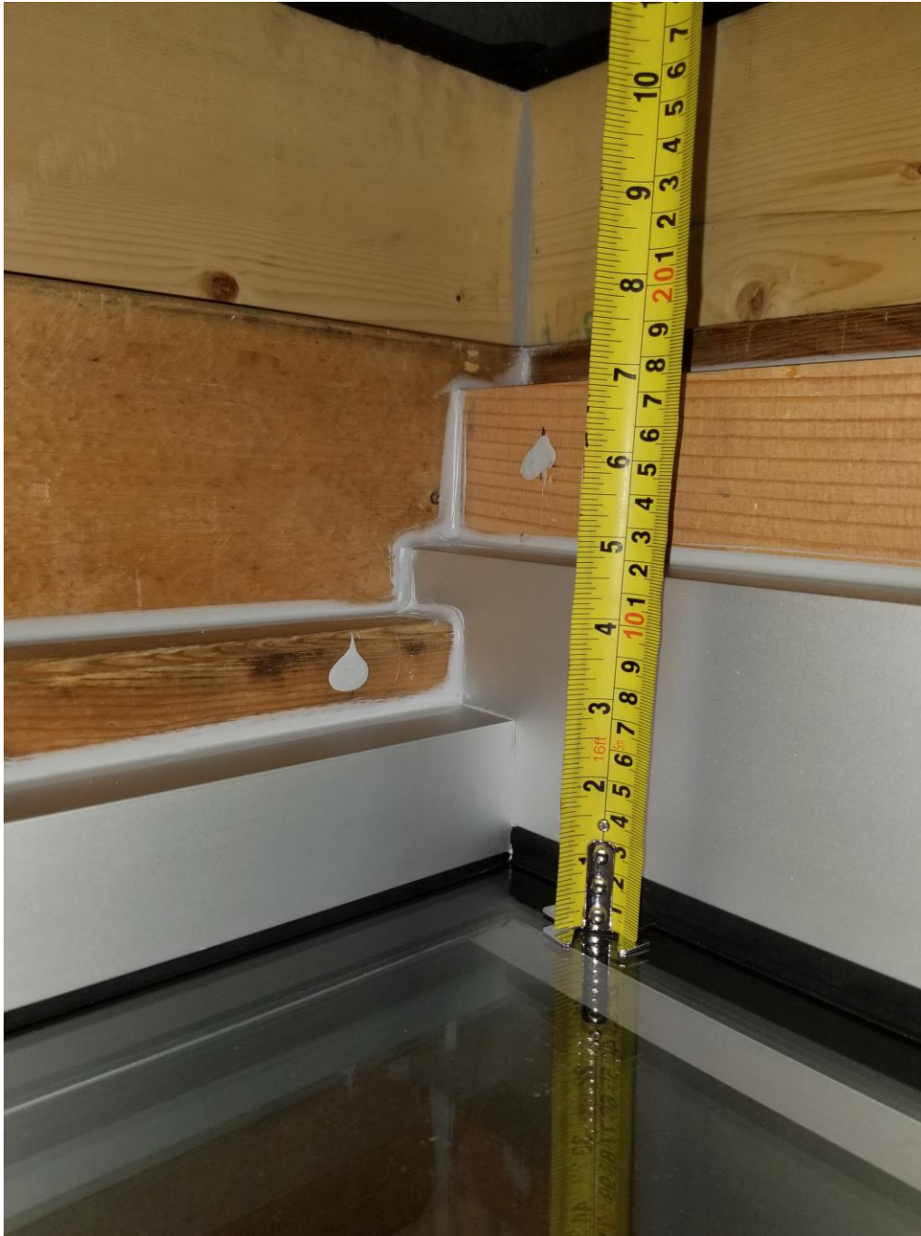
Figure 7: Top interior corner and sealant.
