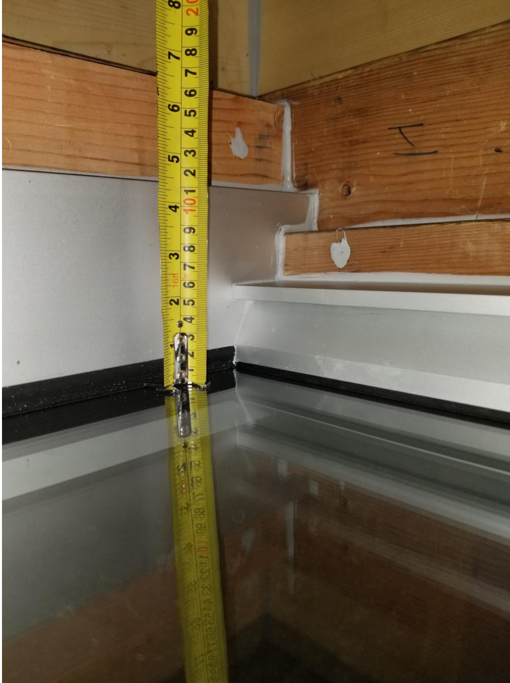
Figure 6: Bottom interior corner and sealant.
